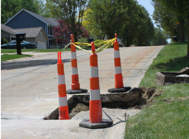
A part of our sewer maintenance program includes rebuilding catch basins and pipe repairs.
