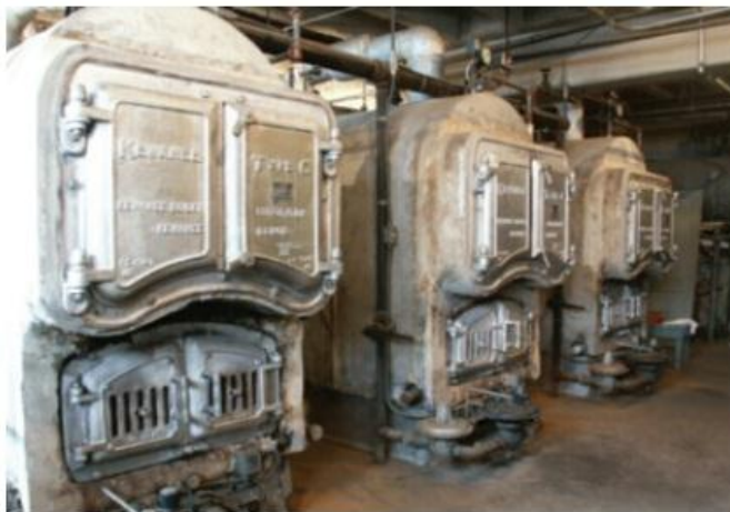
Gas boilers like these vintage 1930 Kewanees still heat some city-owned buildings. Besides the environmental pollution and high energy cost to operate, cities usually don't have money for replacements. An ingenious solution is being implemented by the nonprofit Emerald Cities Cleveland.
